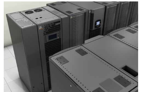
Liebert eXM adjacent to the wall
